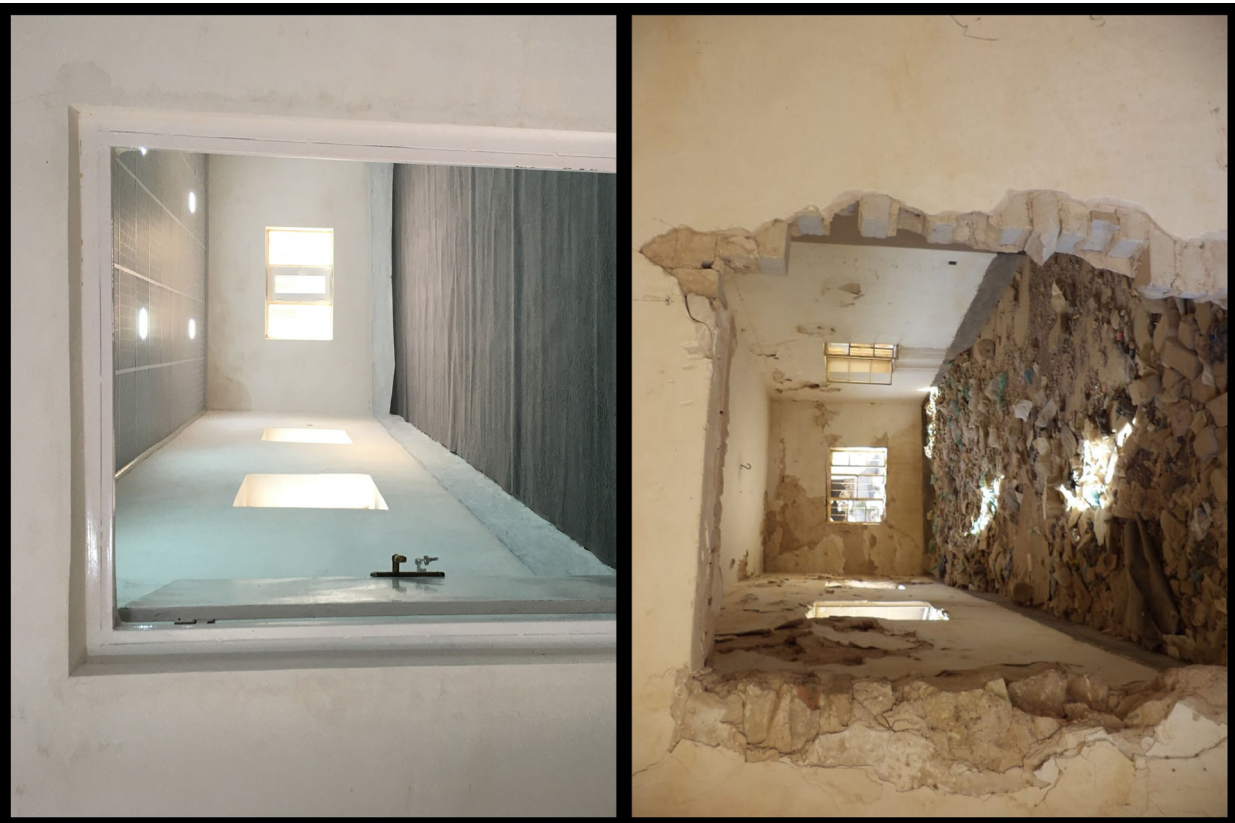
Fig. B1.16: The office room on the north wing's second storey, before and after restoration. Photos by Akam Omar Ahmed Al-Qaradaghi.
