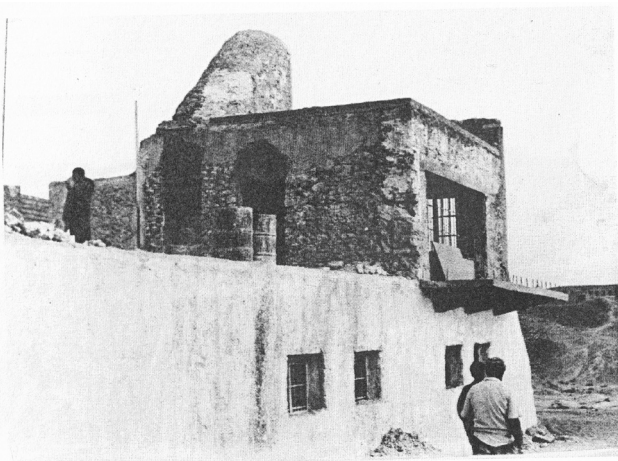
Fig. B4.6: View from the river bank onto the house's northeastern corner in 1978, where the construction of the balcony is in progress. Photo by Mr Muthhir for SBAH Sherqat; reproduced from Jarjis 2020, 75.
