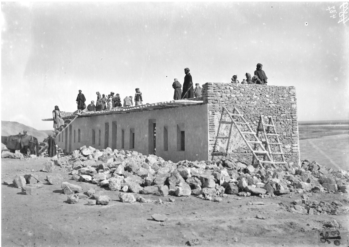
Fig. B2.3: Construction of the east wing of the expedition house in 1903. Bab Ph 487 (© SMB, VAM, DOG; photo by Robert Koldewey).
