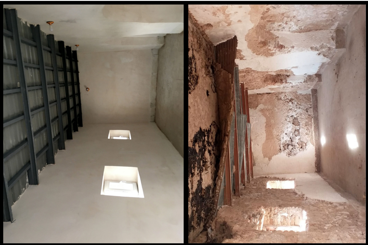
Fig. B1.12: Inside the storage room in the south wing, before and after restoration. Photos by Akam Omar Ahmed Al-Qaradaghi.
