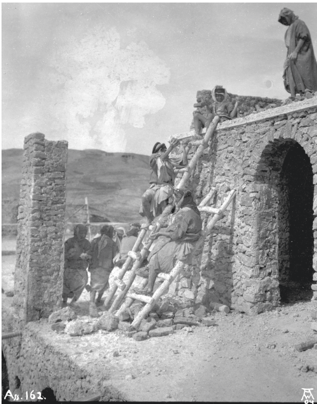
Fig. B2.9: Construction of the living rooms in the north wing. Ass Ph 162, taken on 2 March 1904 (© SMB, VAM, DOG; photo by Walter Andrae).
