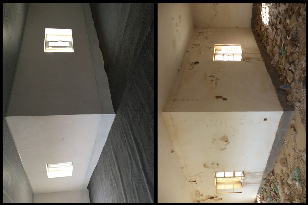
Fig. B1.17: Inside the office room on the north wing's second storey, before and after restoration. Photos by Akam Omar Ahmed Al-Qaradaghi.
