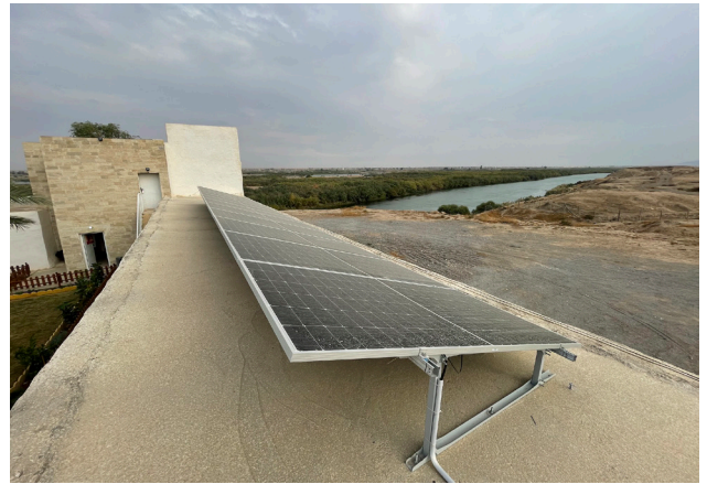
Fig. B5.8: The solar panels installed on the roof of the south wing, with a view of the two-storey part of the building housing the SBAH staff. Photo by Andrea Squitieri.
