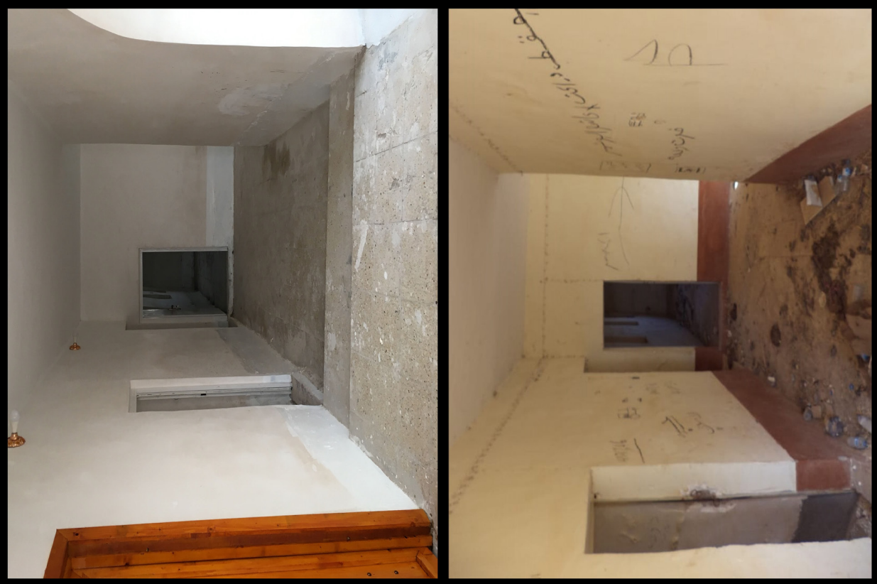
Fig. B1.13: The ground-floor corridor of the north wing, before and after restoration. Photos by Akam Omar Ahmed Al-Qaradaghi.
