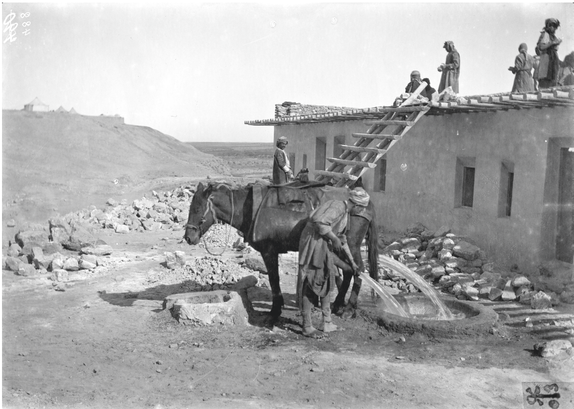
Fig. B2.4: Preparing building materials at the construction site of the expedition house in 1903. Bab Ph 488 (© SMB, VAM, DOG; photo by Robert Koldewey).
