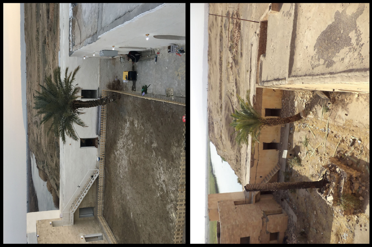
Fig. B1.9: The courtyard as seen from the roof of the north wing, before and after restoration. Photos by Akam Omar Ahmed Al-Qaradaghi.
