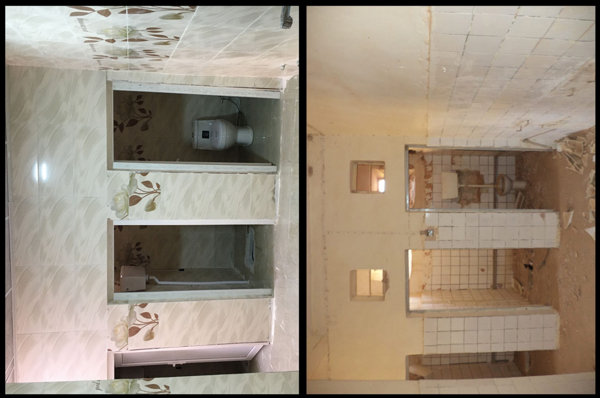
Fig. B1.14: The bathroom on the north wing's ground floor, before and after restoration. Photos by Akam Omar Ahmed Al-Qaradaghi.
