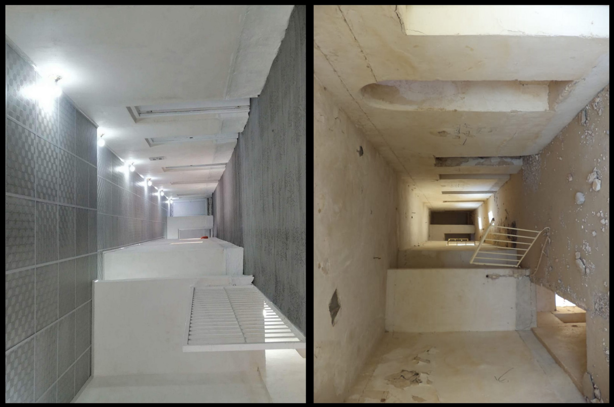
Fig. B1.15: The second-floor corridor of the north wing, before and after restoration. Photos by Akam Omar Ahmed Al-Qaradaghi.
