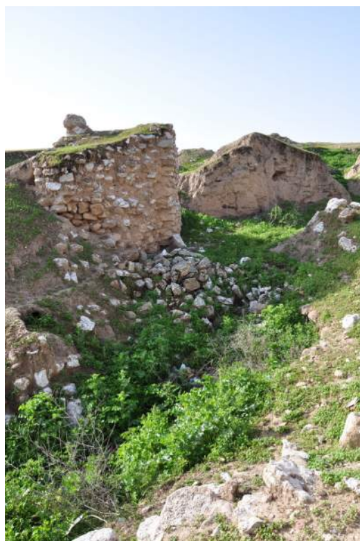
Fig. B1.10: Damage caused by rapid runoff during heavy rainfall. Photo by Eileen Eckmeier.
