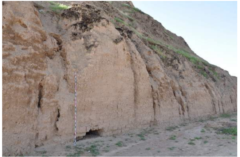
Fig. B1.7: Erosion at the base of the ziggurat. Photo by Eileen Eckmeier.
