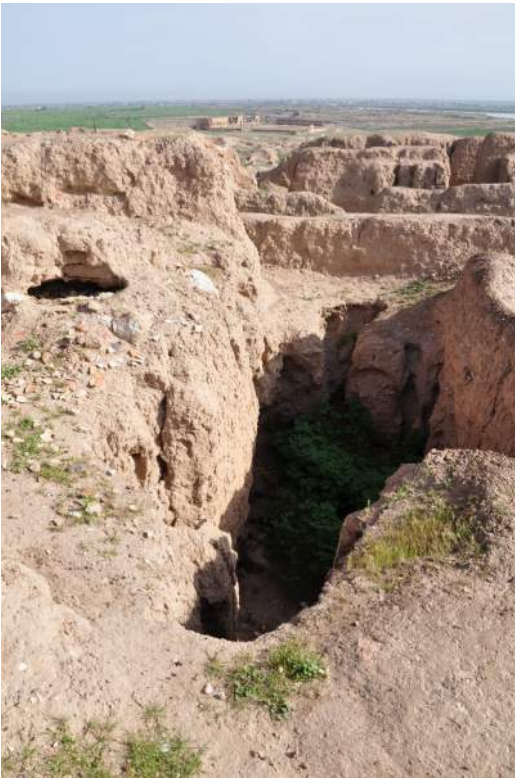
Fig. B1.13: Damage caused by rapid runoff during heavy rainfall. Photo by Eileen Eckmeier.
