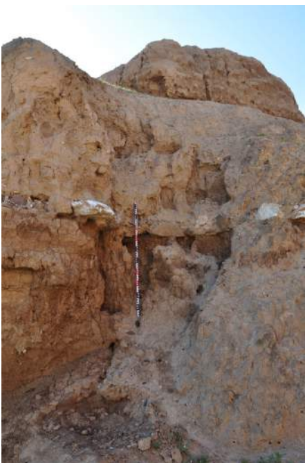
Fig. B1.20: Erosion along the city walls. Photo by Eileen Eckmeier.
