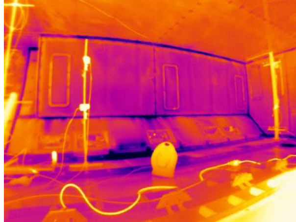
Figure 11: Thermal image showing leakages at the seam between the vertical and inclined liner.
